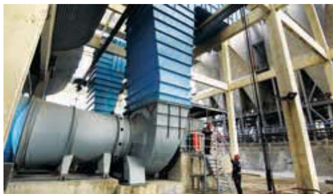
Howden engineers attend a Variax® axial flow boiler draught fan on a coal fired power station
